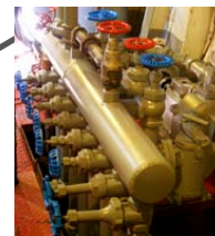
Water manifold, pump and pump motor—motor identified as a General Electric 1942 model.
